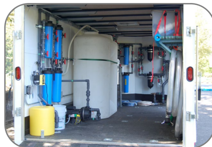
Seven Mobile Water Treatment Systems: Beaverton, Clackamas River Water, Lake Oswego, Portland Water Bureau., Gresham, Milwaukie, and South Fork Water Board
